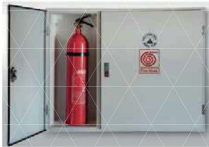
► Extinguisher Fire Box
